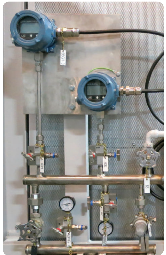
Seal Pressure Monitoring
