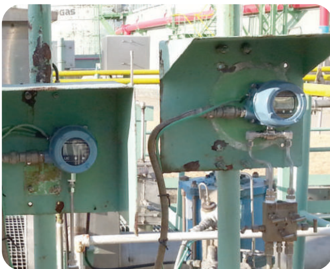
Natural Gas Monitoring
